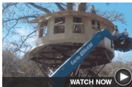
Not Your Childhood Treehouse Watch this fascinating time-lapse film of building the bibliotèque (library) treehouse in Utopia, Texas, where you can stay overnight.
